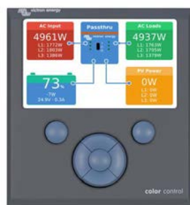
Color Control panel, showing a PV application
